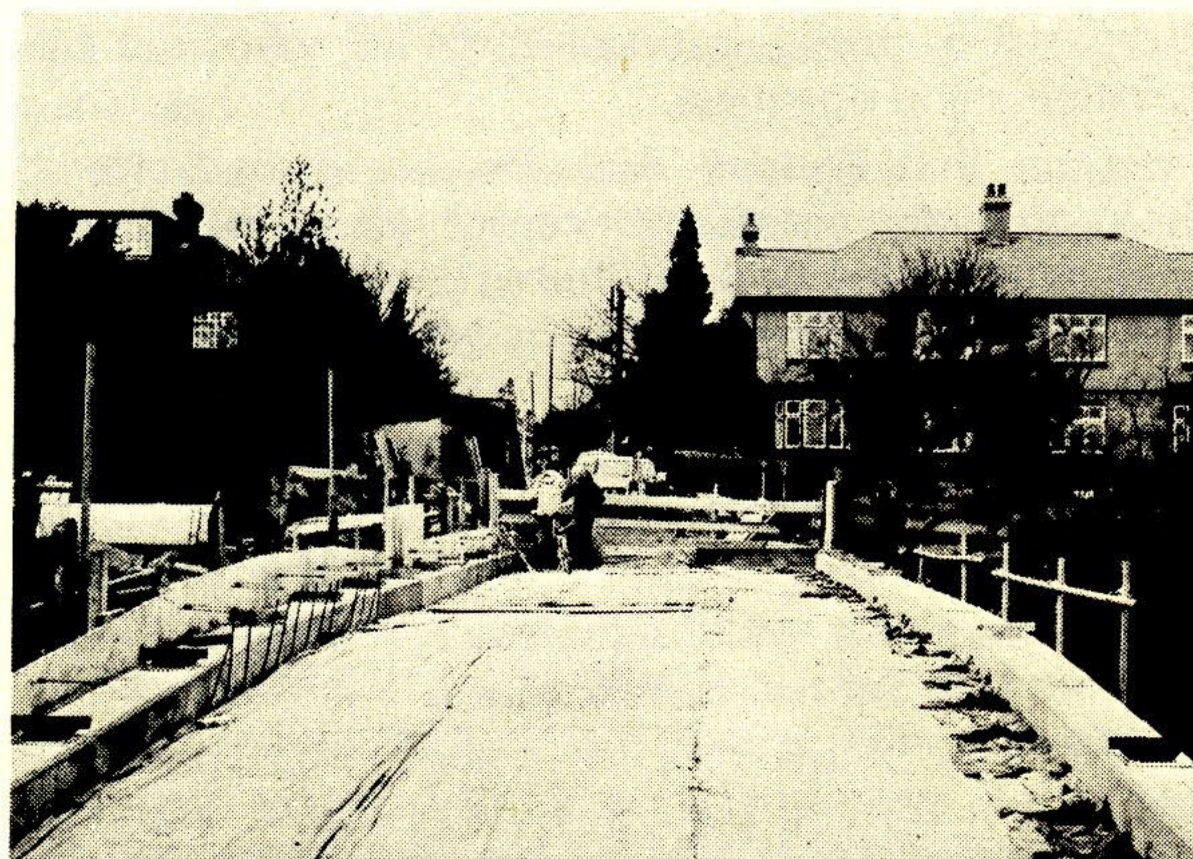
Bumbler Box bridge (off Woodcroft Road). Repairs in progress May, 1976. Now completed.
