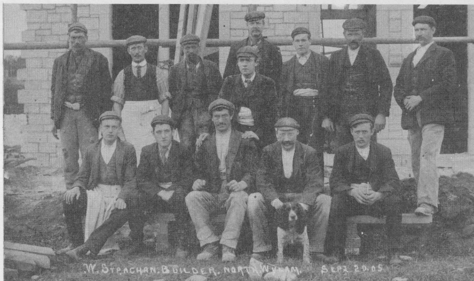
A very fine photograph of W. Strachan's team of 13 men and boys (plus dog), posing proudly in front of No. 21 Stephenson Terrace, under construction on 20th September, 1905. Does anyone recognise any of these men as being former Wylam residents?
