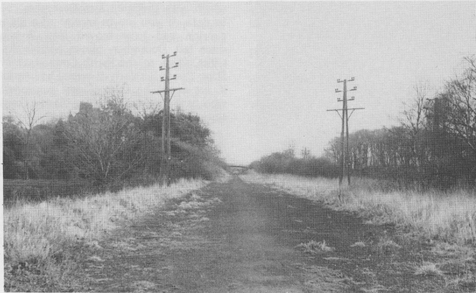
These two electricity poles alongside the old railway track should be removed when NEEB replace the overhead line.
