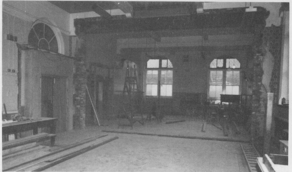
Work in progress, transforming the two ground floor rooms in the Institute.
