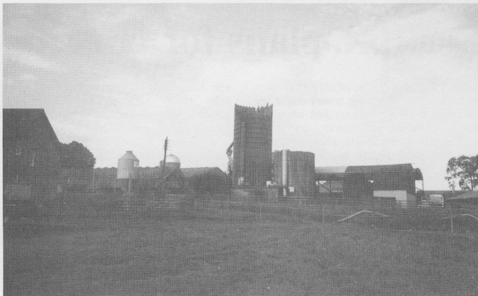
Disappearing landmarks – the two concrete silos at Robert Graham's farm under demolition in July.
