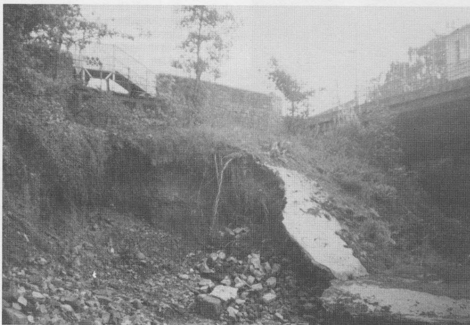
Getting bigger and bigger—the area of erosion in the river bank immediately below the access into the Station car park and next to the bridge. British Rail have now promised that repairs will be carried out this year . . . a stitch in time?
