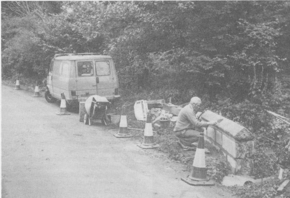
Prompt repairs in progress to the damaged bridge on Blue Bell Lane.
