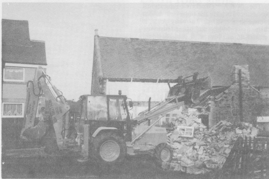
Work in progress to demolish the former caretaker's cottage, the vestry and outbuildings adjoining the Methodist Chapel. Construction of the new building is now underway.
