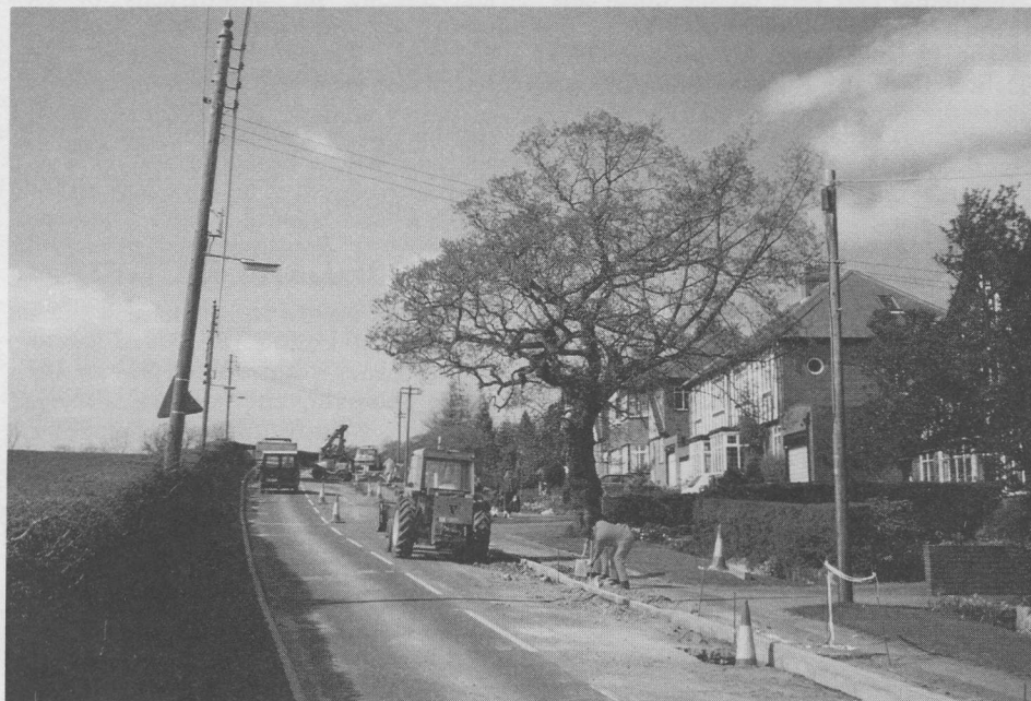
Although the roadworks and temporary traffic lights have effectively reduced the speed of traffic on Holeyn Hall Road over recent weeks, most residents will be pleased that work is nearing completion.
