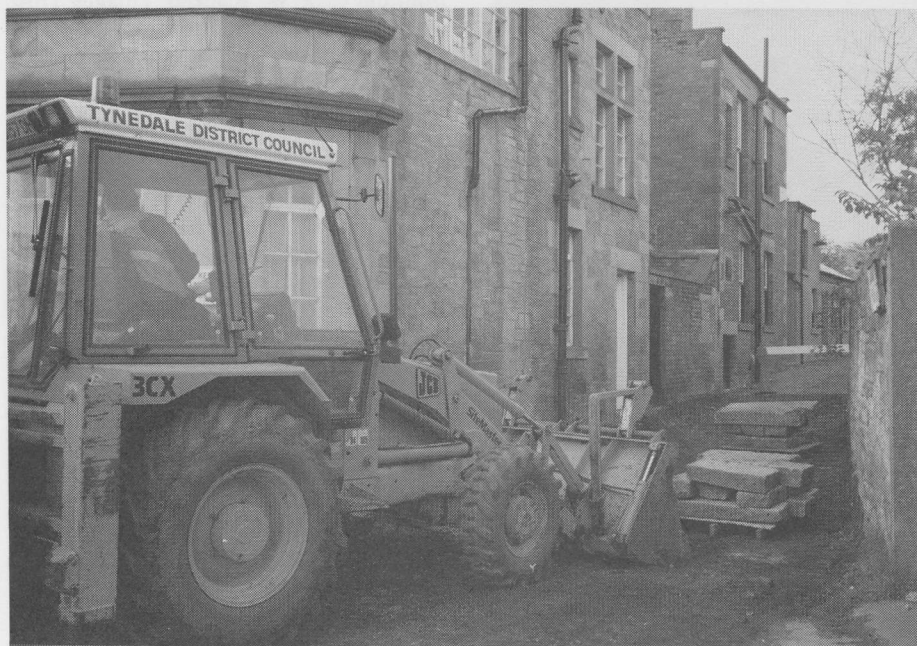
It'll never be the same again! Work in progress by Tynedale on behalf of the Parish Council to complete the resurfacing of Ship Inn Lane. This is probably the first time that it has ever had a proper road surface.
