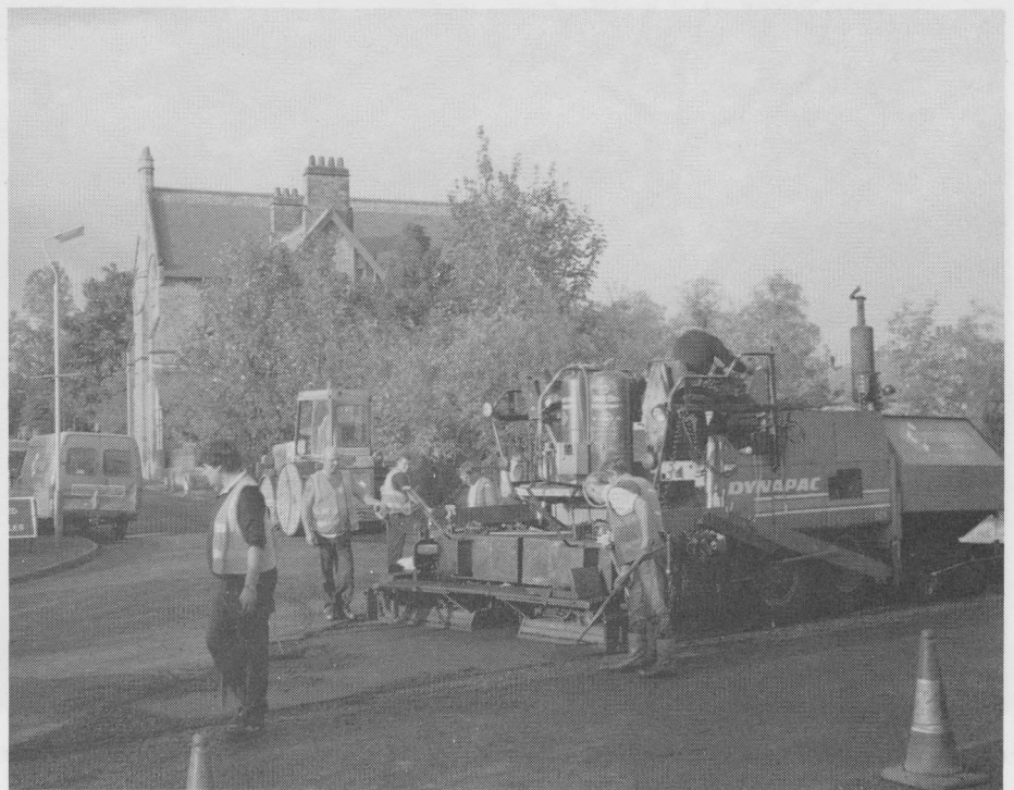
Chaos in a good cause! Contractors busy resurfacing the road junction by the Institute garden - part of the scheme to create a greatly improved surface to Church Road. The next question is which company will be the first to dig it up - gas, electricity, water/sewer or telephone?
