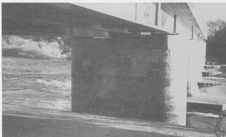
A view under the northern end of the bridge showing the concrete apron sloping down to the edge of the river. A barrier will be erected along the edge of the concrete and more signs displayed in the vicinity.
