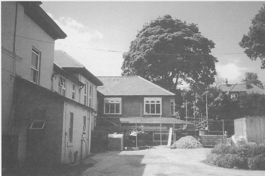
Taken several weeks ago, this picture shows work in progress on the major extensions to the Stanley Burn Residential Home. The new accommodation should be completed shortly and will increase the number of rooms for residents and greatly improve the facilities at the Home.
