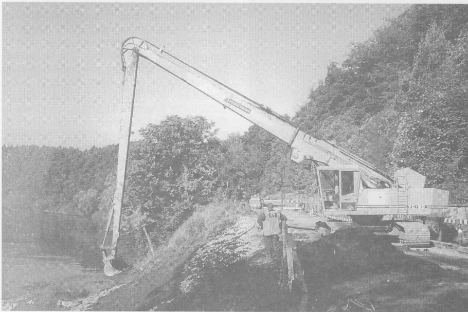
Work on stabilising the riverbank and repairing the Ovingham road was completed by mid October. Contrary to early speculation the soil survey showed that the road-slip was caused by the collapse of an old coal-seam below the road, rather than by river erosion.
