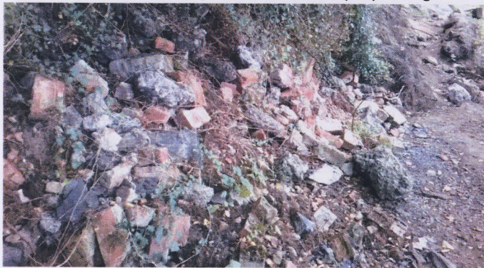
Damaged Riverside path below Tom and Joes
