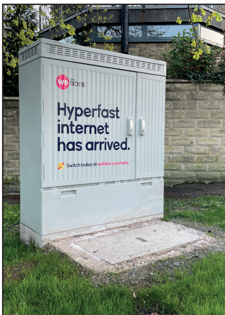
The new We-Fibre cabinet on Woodcroft Road
