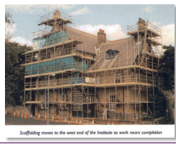
Scaffolding moves to the west end of the Institute as work nears completion
